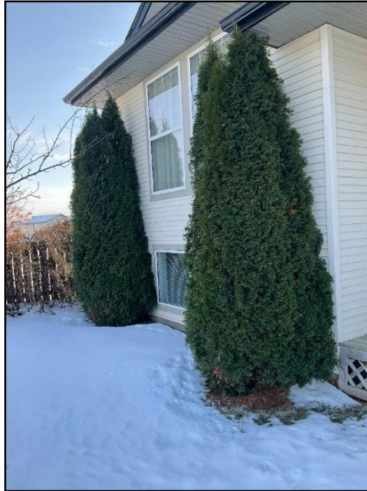
11. Trees or shrubs too close to building
